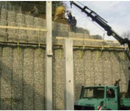
Stabilization of an embankment (height 11 metres) in the direct neighbourhood of a shopping centre in Pegnitz/Bavaria
