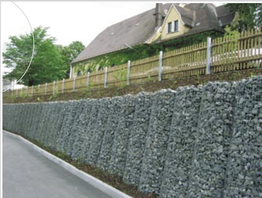
The FERRONDO® slope stabilization (here in inclined arrangement) adapts to the environment harmoniously (left)
