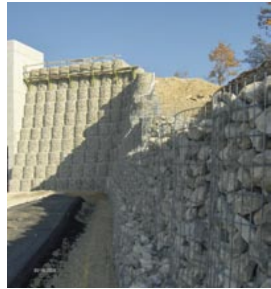
Stabilization wall (height 14 metres) under construction at a company site in Laaber/Bavaria
